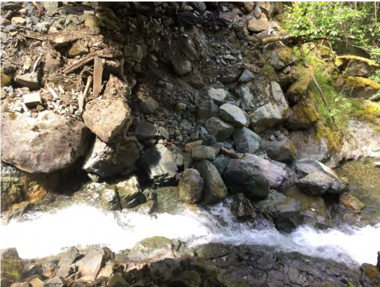
Failed riprap at left bank
